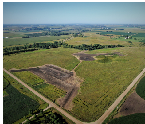
Aerial view of the CREP wetland restoration during construction on the Schaefer's CREP easement.
