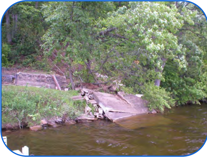
Before Project – Boathouse/Bluff Failure
