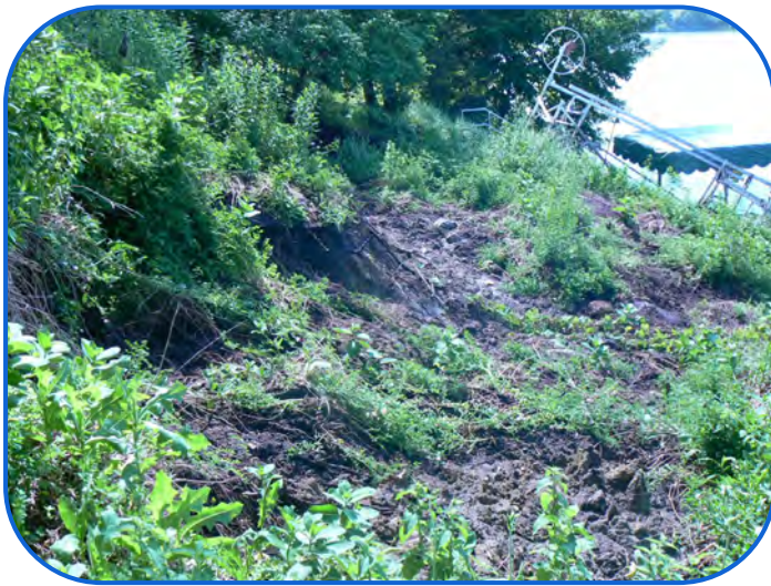
Before Project – Slope Failure
