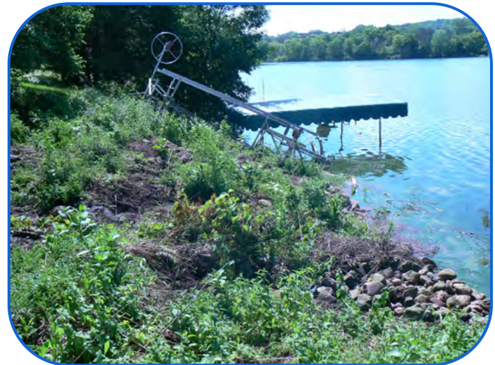
Before Project – Slope Failure
