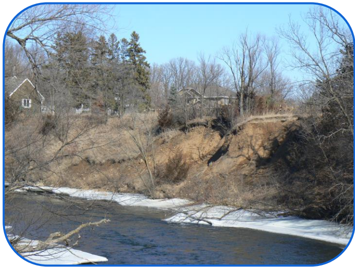
Before Project – Failing Slope
