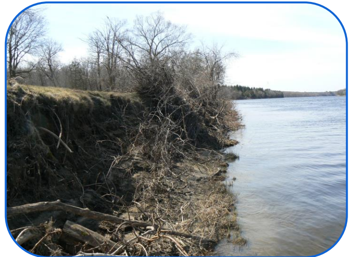
Before Project Streambank Erosion
