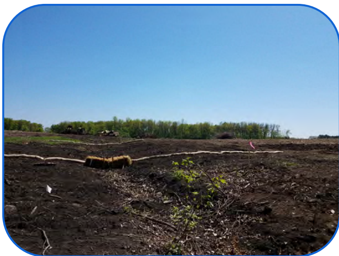
Gully In Field Prior To Project
